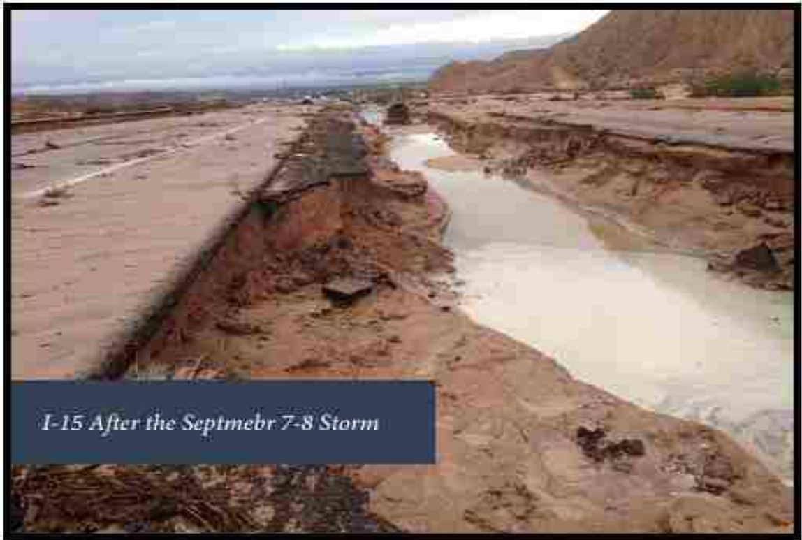
Figure 2.5-3: Photo of a damaged section of I-15 due to the flood events of Sep 07, 2014. (Source: CCRFCD)
