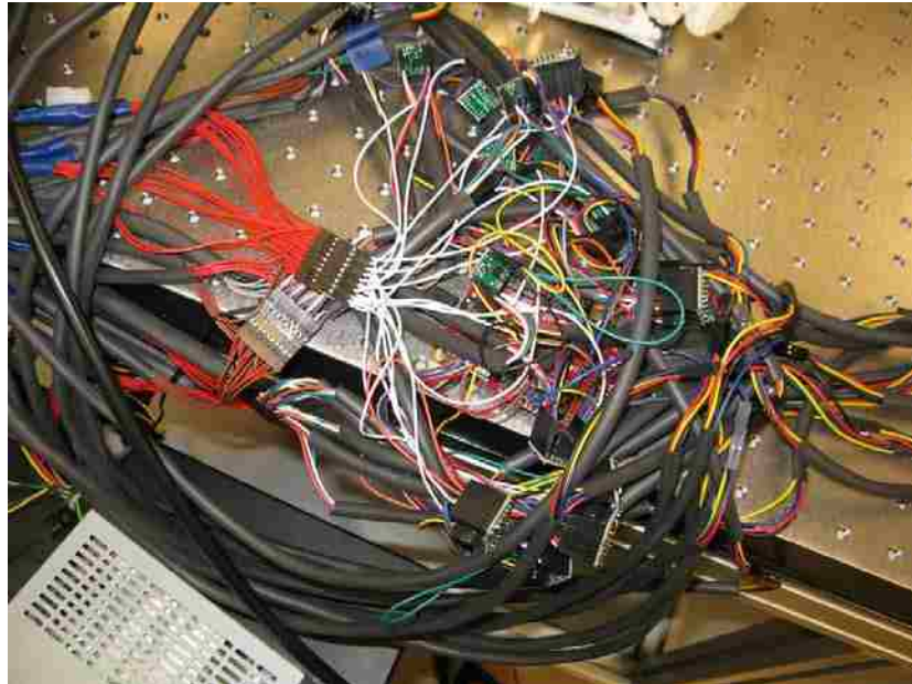
Figure 40: Nest of wires and drivers.
