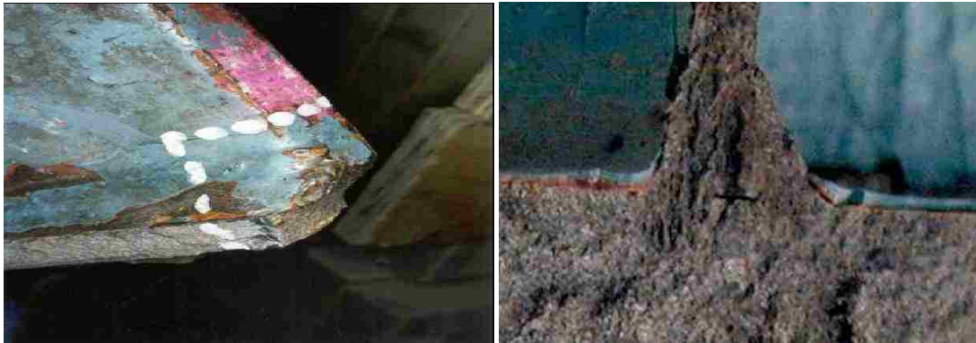
Figure 1.3 Fracture in highly constrained welded plate girders. [8]
