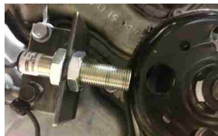
Figure 3. 8 – Laser tachometer aimed at water pump.
