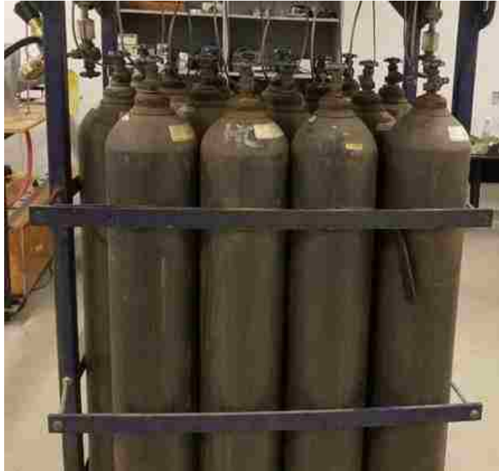
Figure 3.10: Pressurized N 2 tanks
