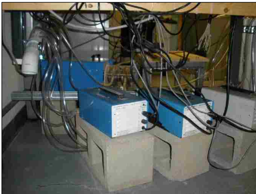
Figure 3.10 Pumps and plumbing of the evacuation system used to empty collection vessels
