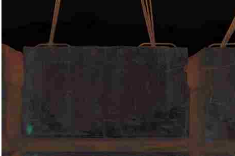
Figure 1-6: Effect of Combined ASR and DEF on Precast Beam (Skalny et al. 2002)
