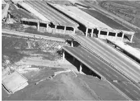
Figure 2-4 Superstructure failure due to unseating (Andrawes and DesRoche 2005).
