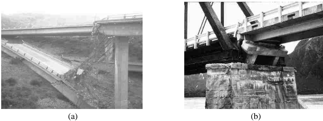
Figure 2-3 Damage due to seismic pounding: (a) In-span hinge seat failure causing unseating (Muthukumar 2003), and (b) near-collapse of Copper River railroad bridge in 1964 Alaskan Earthquake (United States Geological Survey [USGS]).
