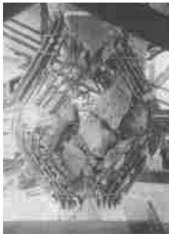
Figure 2-20 Shear failure of La Cienega-Venice Undercrossing Collector Distributor 36 possibly caused by axial tension (Papazoglou and Elnashai 1996).
