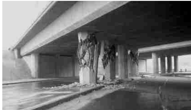
Figure 2-18 Column failure of Foothill Boulevard Undercrossing caused by effects of skewed superstructure (Earthquake Engineering Research Center, University of California-Berkeley).
