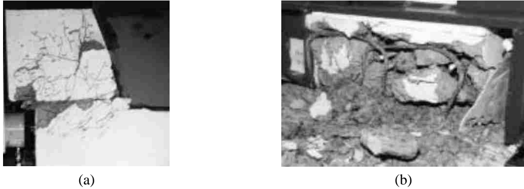
Figure 2-7 Failure of shear keys: (a) exterior key, and (b) interior key (Megally et al. 2002).
