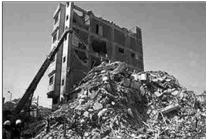
Figure 1-3 Collapse of clothing factory in Alexandria, Egypt ( Factory fire kills 15 in egypt.2000 )
