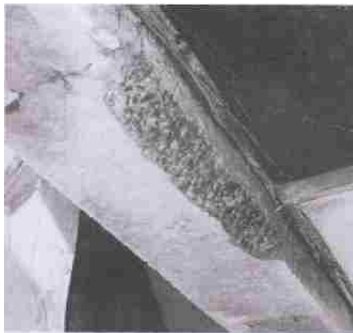
Figure 2-8 Spalling at corner of concrete beam subjected to fire (Buchanan, 2001)
