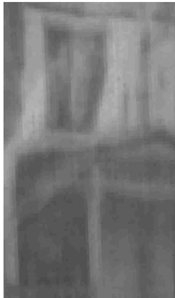
(c) A close-up of a heavily distorted window.
