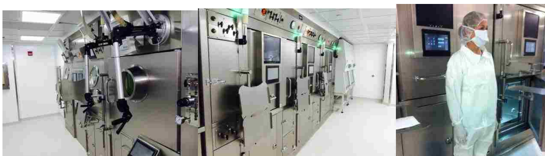
Figure 15. images of ISO 7 GMP area at WUSM Cyclotron Facility and Nuclear Pharmacy
