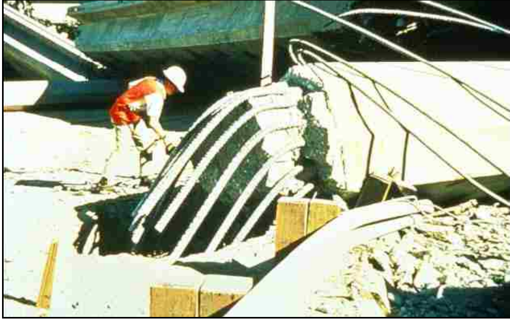
Figure 2.8 Pullout failure, 1971 San Fernando earthquake (Caltrans, 2003)
