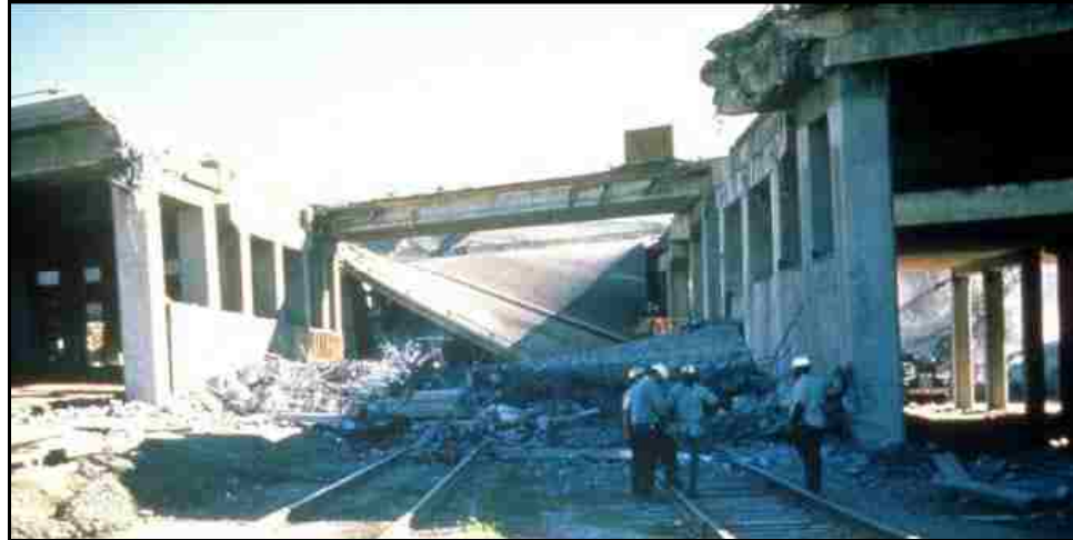
Figure 2.2 Spans slipped off narrow support seats, 1971 San Fernando earthquake (Caltrans, 2003)
