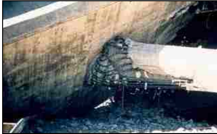
Figure 2.5 Confinement failure at column top (Caltrans, 2003)
