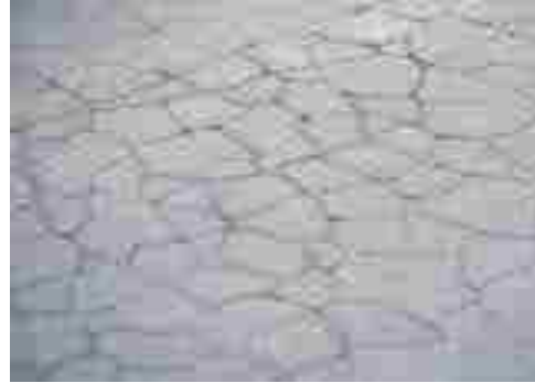
Map or pattern cracks
