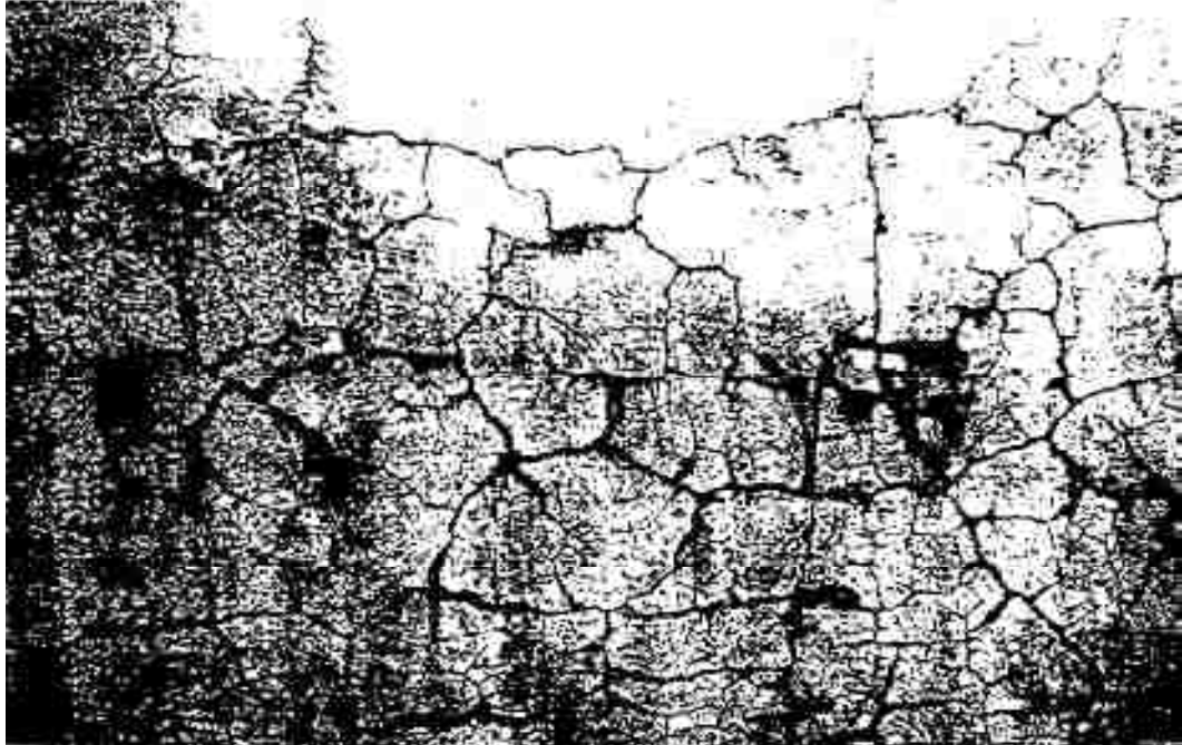
Figure 1.3: ASR cracks in the concrete of Hoover Dam (Hobbs, 1988)
