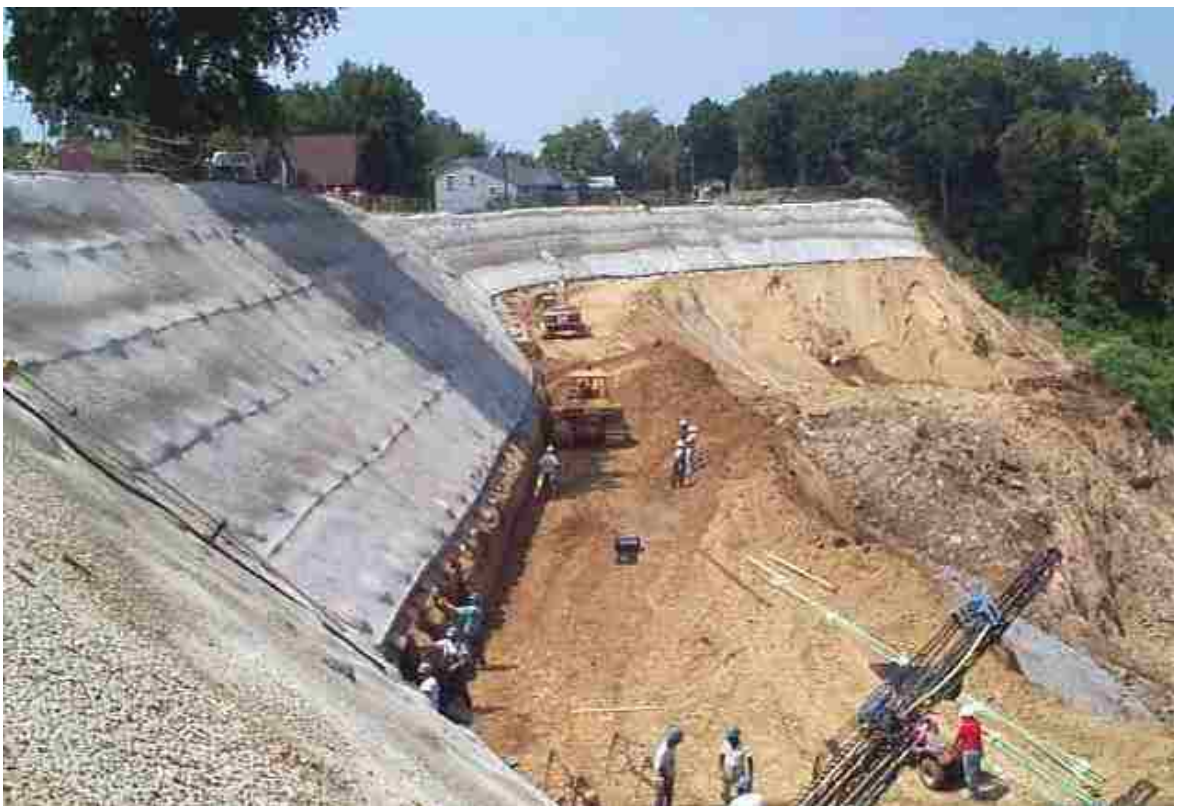
Figure 6.1: An example showing the use of steel rods and concrete to stabilise a hillslope.
