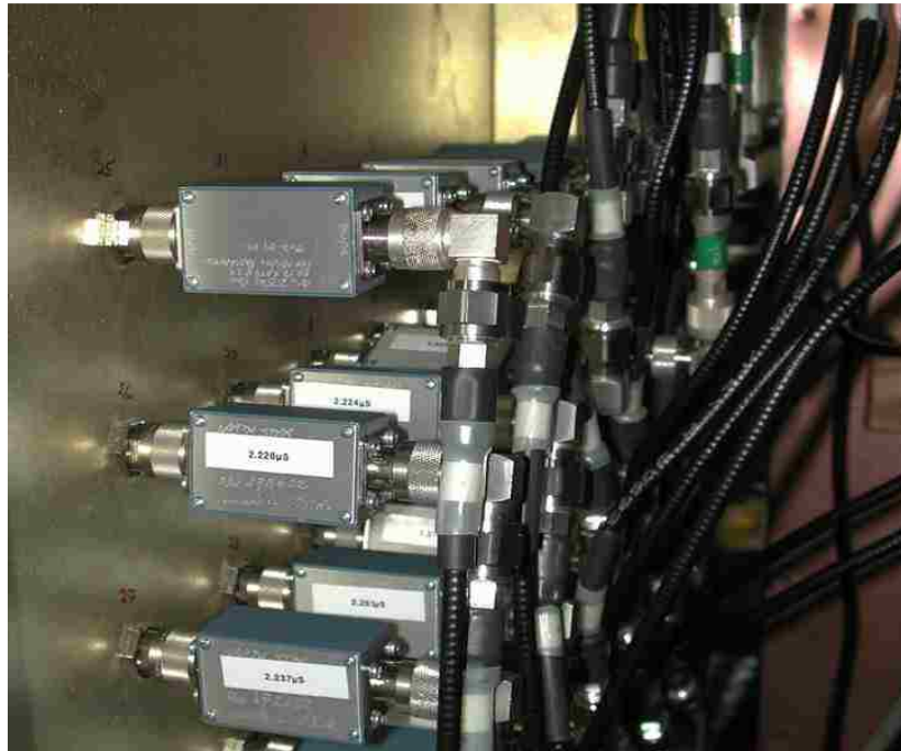
Figure 3.16: RC passive integrators. There is a single calibrated integrator for each of the 24 B-dot signals.
