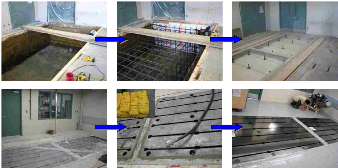
Figure 3-1 Dynamometer Test Bed Preparation
