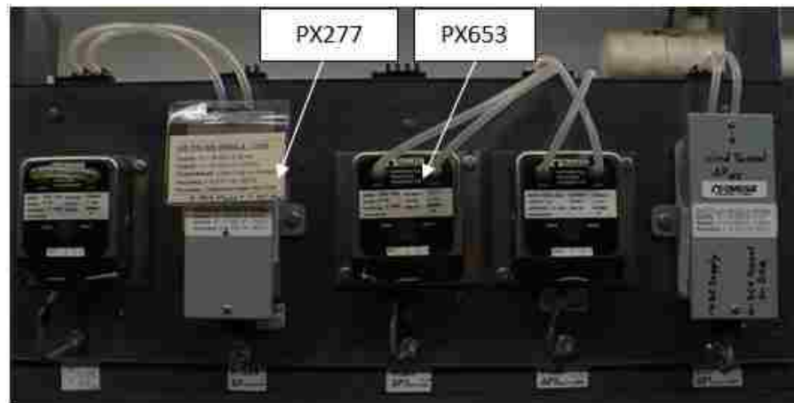
Figure-4. 14: Differential Pressure Transducers (DPTD)
