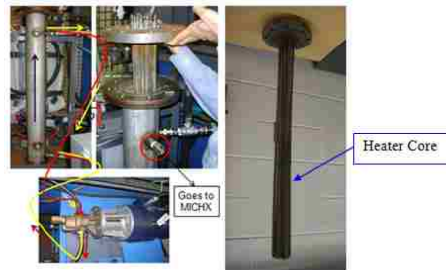
Figure-4. 3: Recirculation Pump and Heater Element
