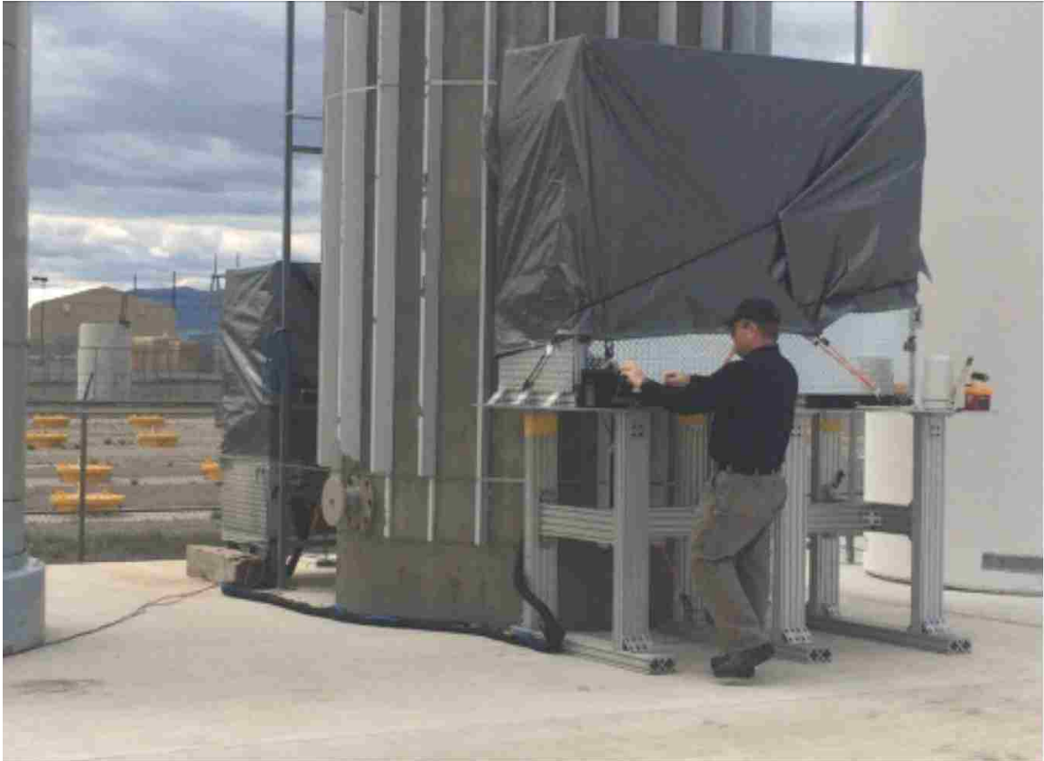
Figure 4.14: Both supermodules in new weatherproof containers around the MC-10.
