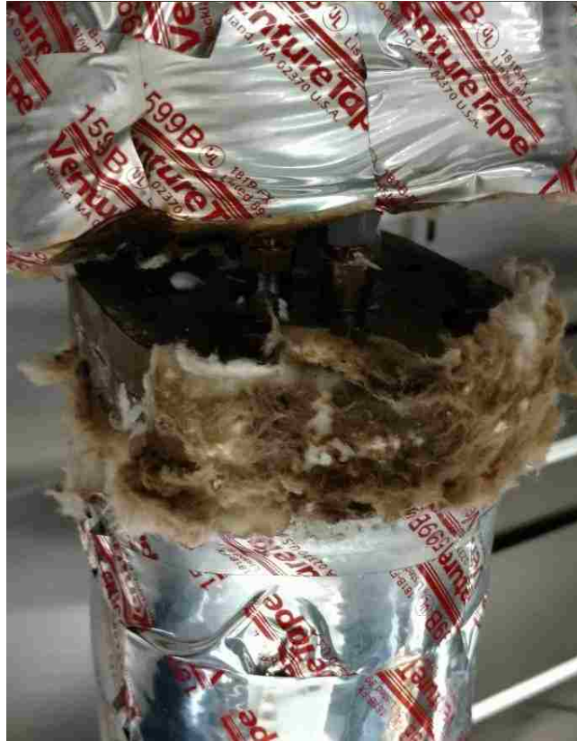
Figure 3-26 Salt leakage around expansion tank gasket
