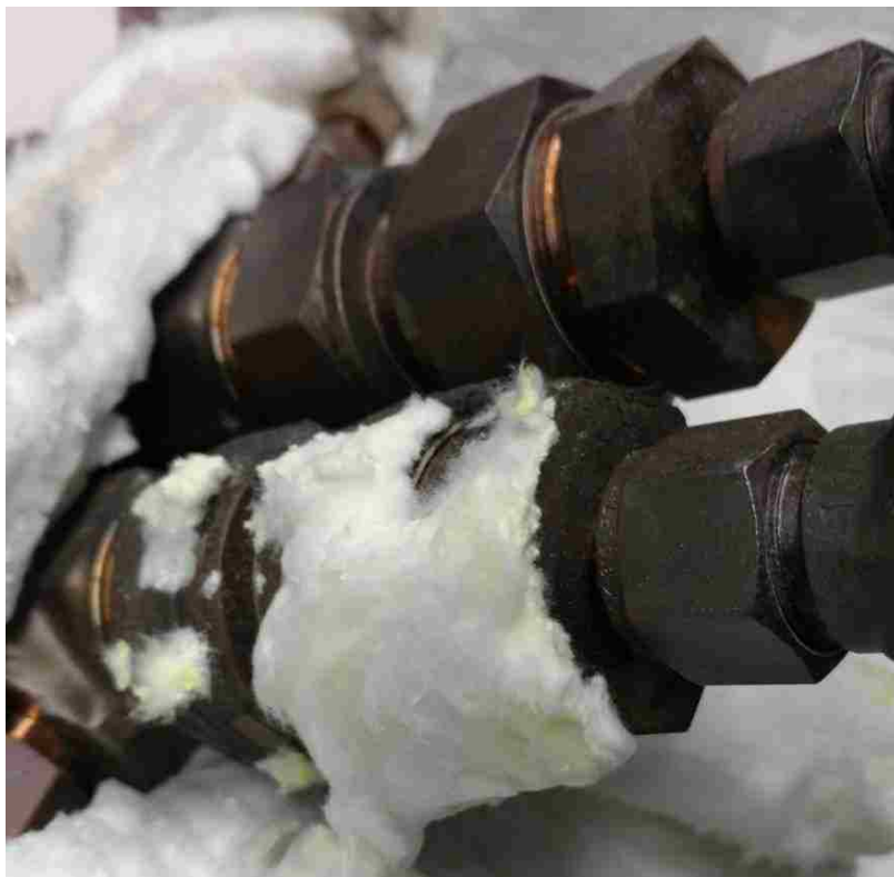
Figure 3-28 Pump outlet loop leg salt leak site
