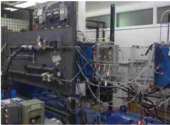
v. Instrumentation and System Insulation-1
