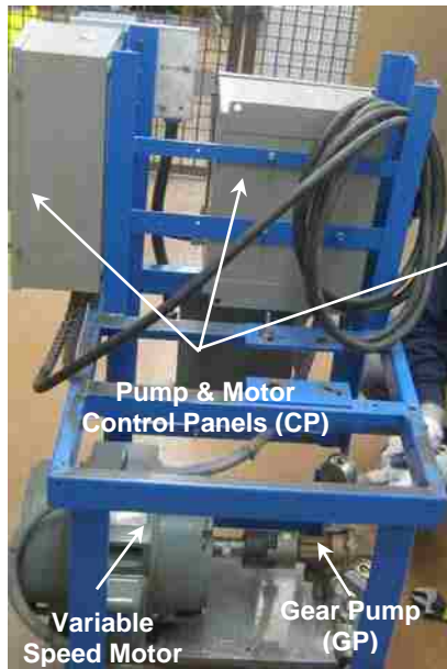
m. Pump-Motor Cart Unit Assembly & Fitting
