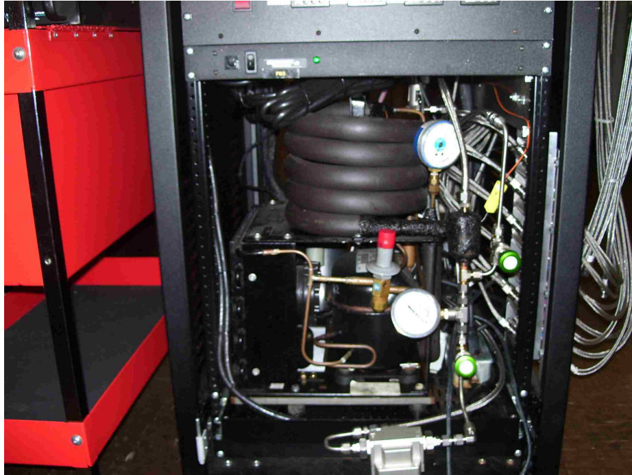
Figure 3.4: Gas Chiller used in CAI Sampling System
