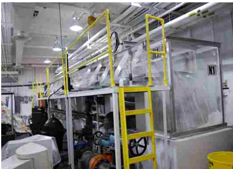
Figure 3.2: The open-channel flume in operation.
