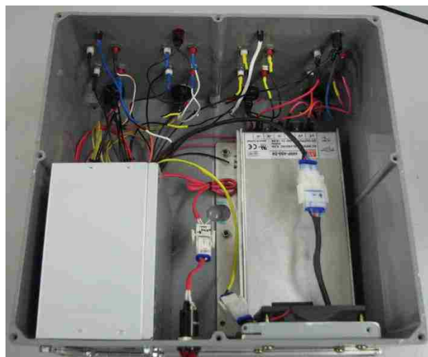
Figure 4.16: Power Supply Inside View
