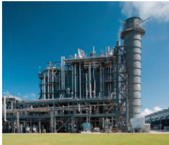
Figure 2.1: OUTSIDE VIEW OF HEAT RECOVERY STEAM GENERATOR
