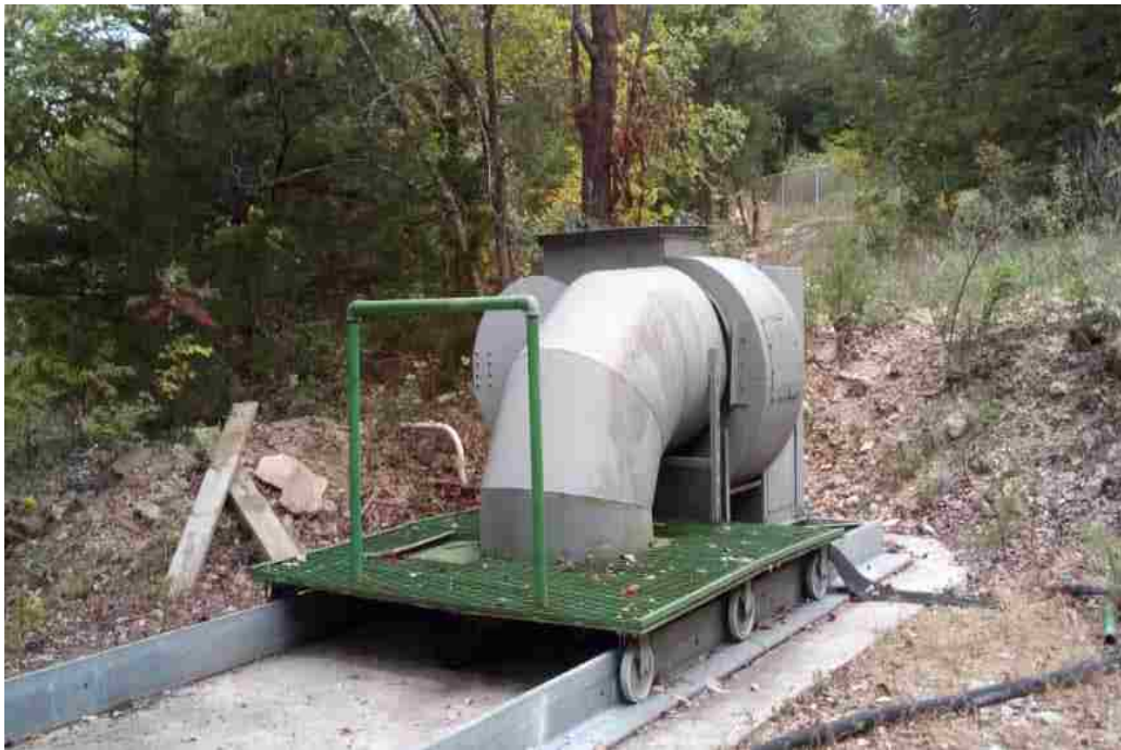
Figure 5.3. Illustration of exhaust fan at the surface
