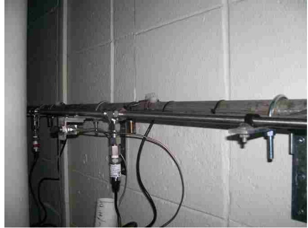
Fig. 3.9. 0.5 and 1 inch stainless steel pipes
