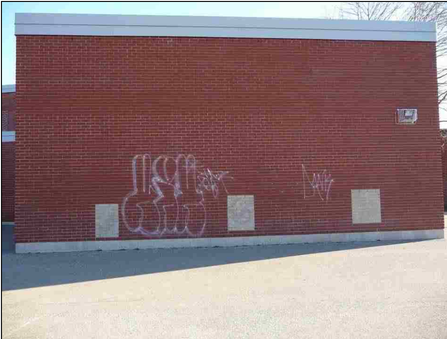
Figure 75. ES-10: Evidence of vandalism along an exterior wall of the school building.
