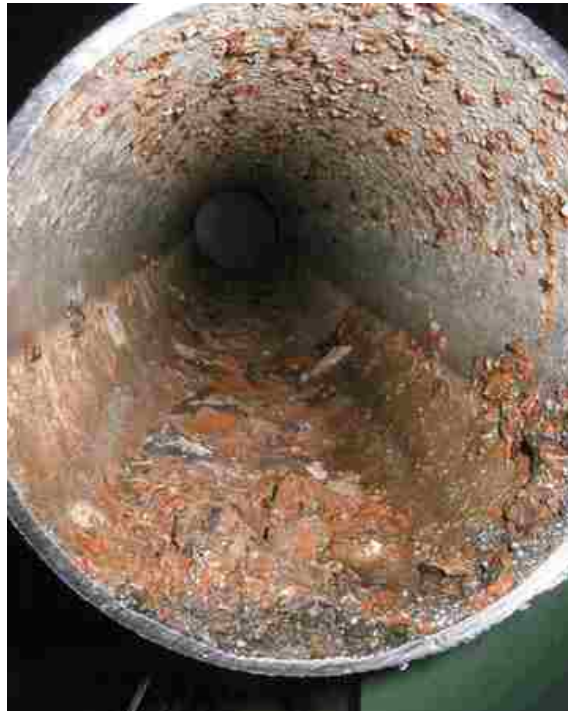
Figure 1.1: Internal corrosion of a typical pipework section
