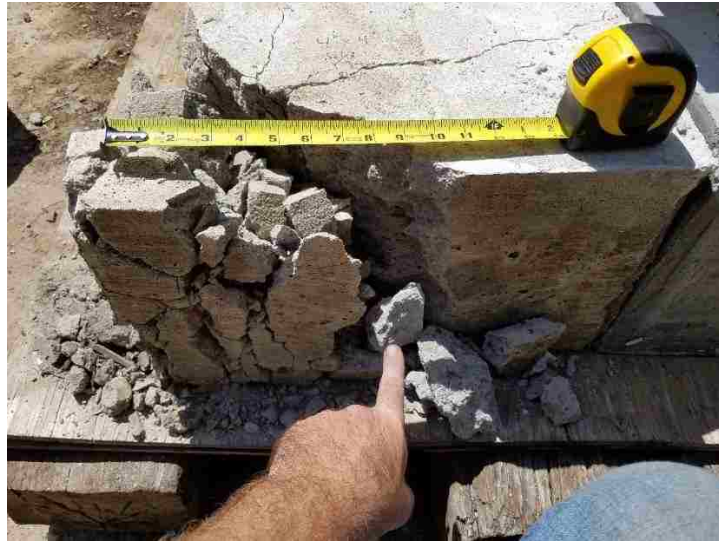
Figure 10 Side Breakage Test 5
