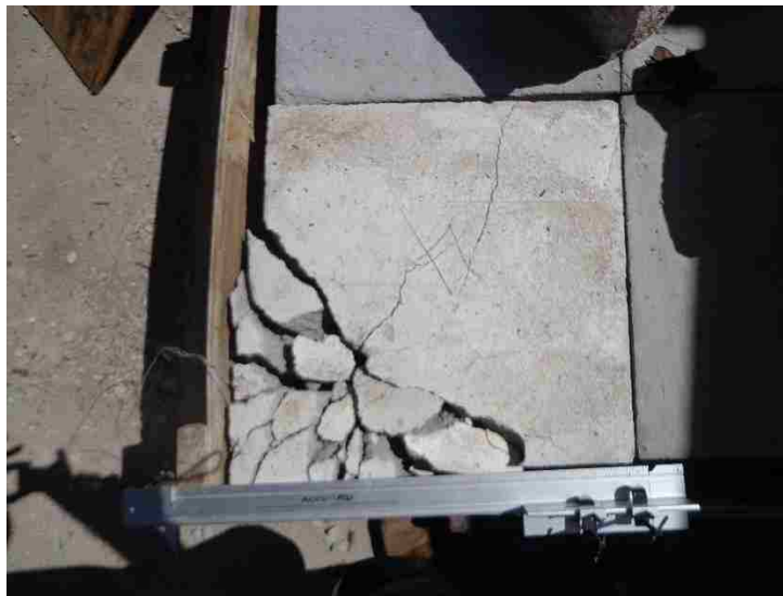
Figure 1 Surface Breakage Test 1
