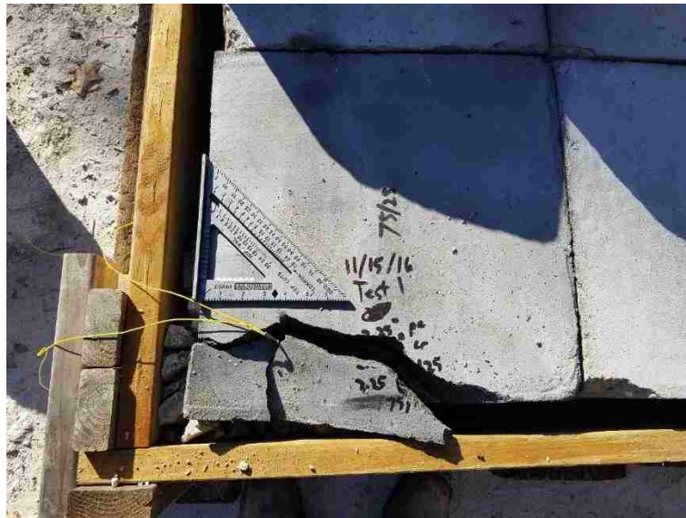
Figure 23 Surface Breakage Test 15
