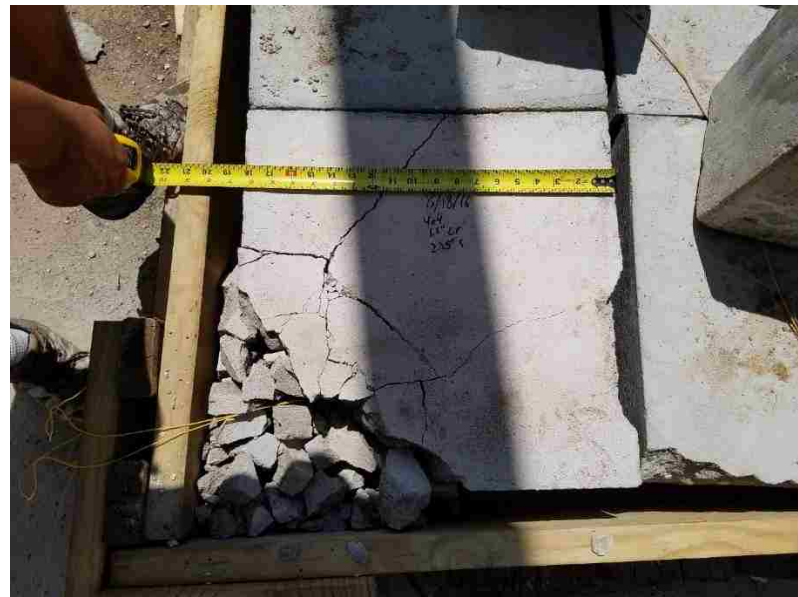
Figure 17 Surface Breakage Test 9
