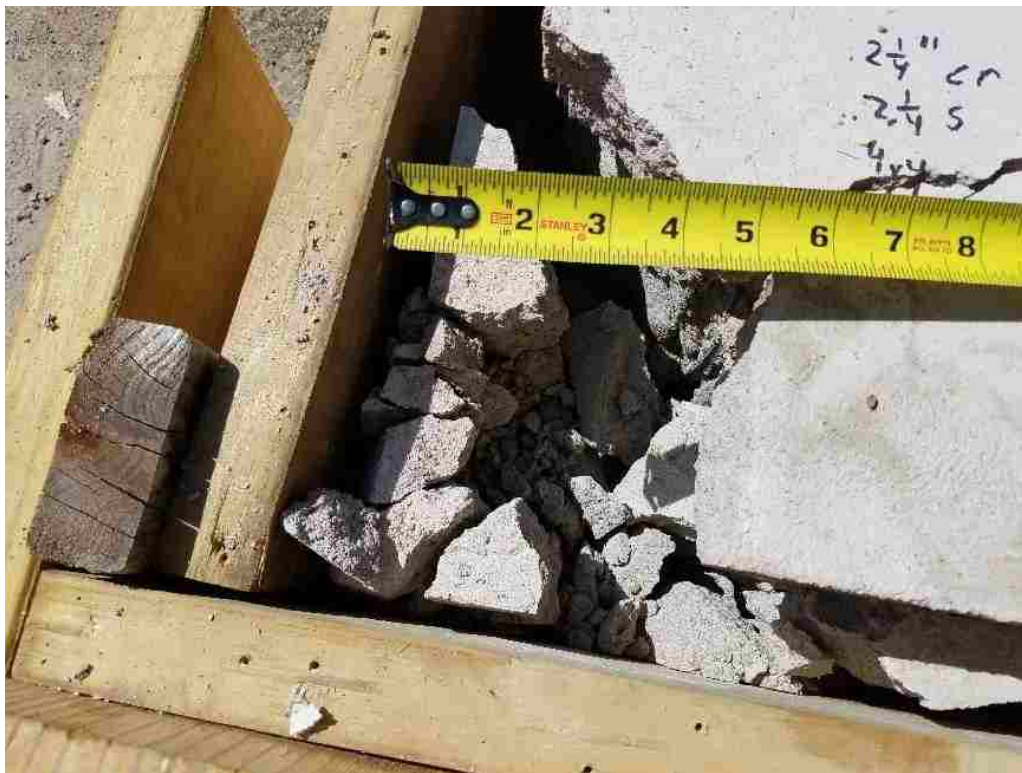
Figure 5.5. Breakage of Substrate, Test 7 8/18/16
