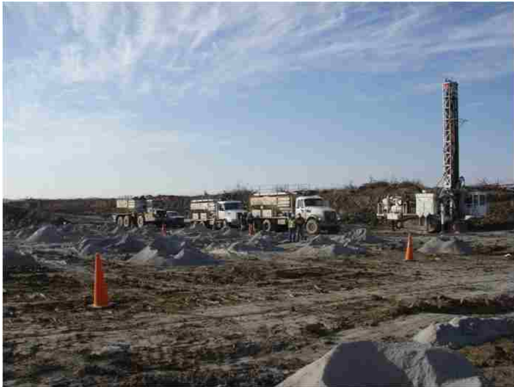
Figure 2.5. Grid of blastholes filled with ANFO. Note gray mounds denote excess nitrogenous chemical around each blasthole.
