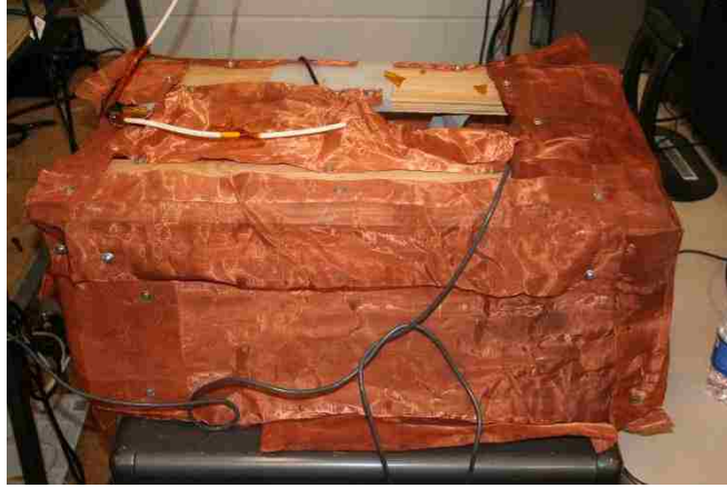
Figure B.3: The faraday cage is used to keep the high voltage transformer from picking up ambient noise.
