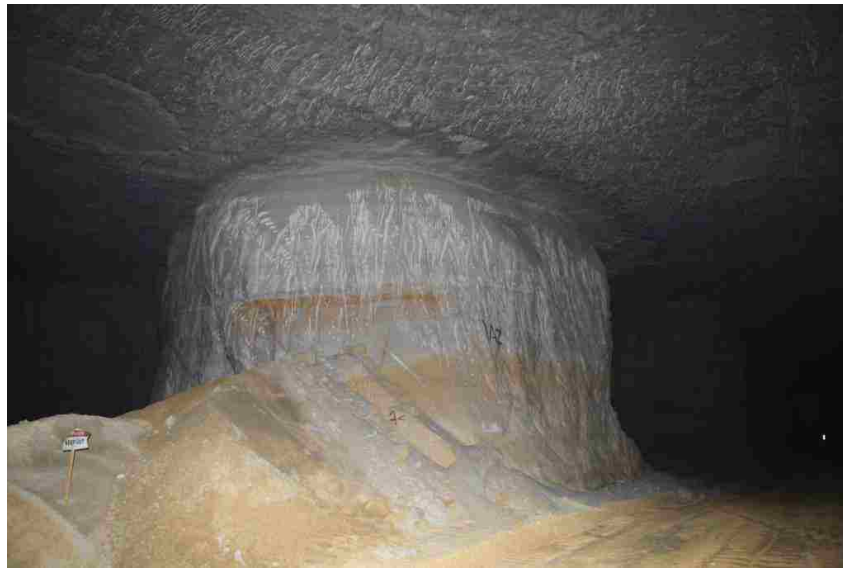
Figure 4.16. Pinch-out failure, severe fractures developed between pillars and cap rock roof.
