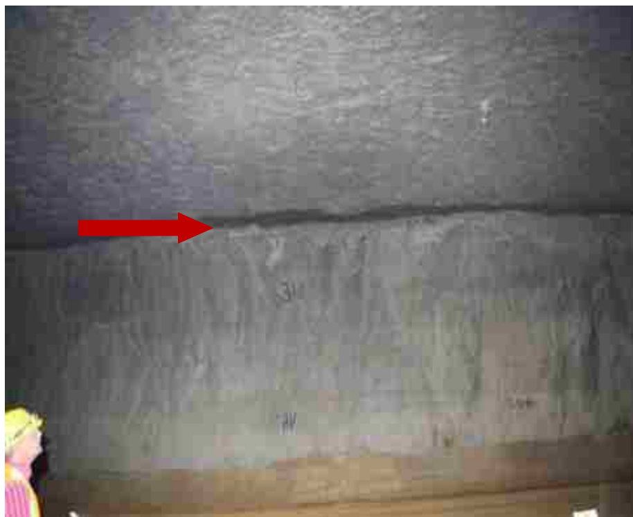
Figure 1.3. A pinch- out failure in the Pattison Mine
