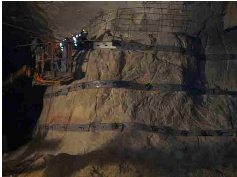
Figure 4.44. An attempt to stop a progressive pillar failure by rockbolting and steel stripping.
