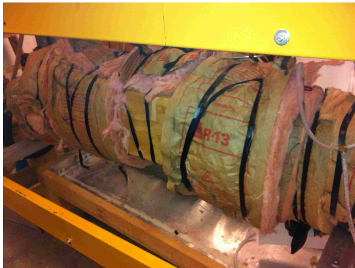
Figure 3.13: Fully insulated liquid test section.
