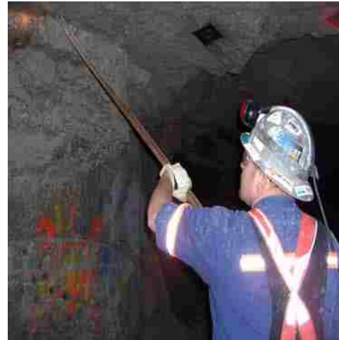
Figure 2.3. Scaling in a Mine.
