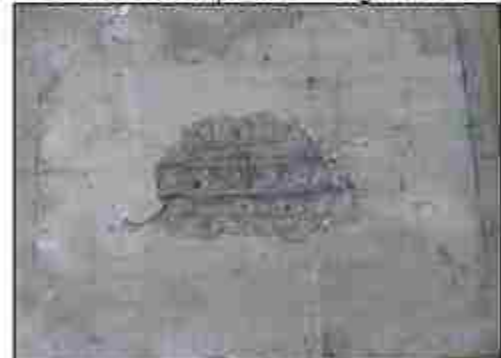
Panel 4 rear surface after explosion - Heavy scabbing, reinforcing bars exposed. - Cavity approximately 480 mm x 300 mm, with a maximum depth of 50 mm (1/2 section depth).
