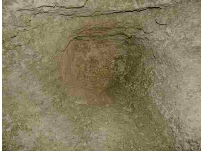
Figure 4.1. Typical Baseline Relief Hole Round (This picture of Test 10's results illustrates the uniform profile at the back of the cut, containing no craters or bootlegs)
