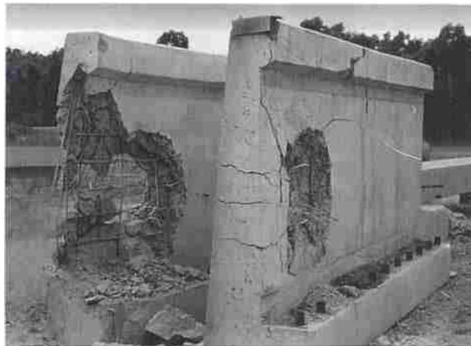
Figure 1.1: Reinforced concrete after EFP impact.(2)
