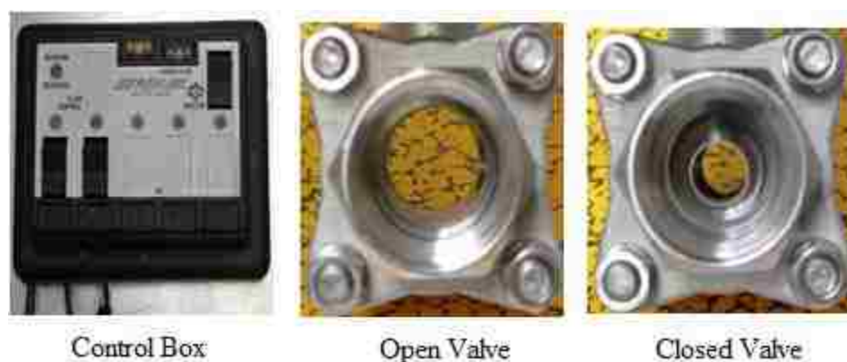
Fig.6. Pneumatic Flow Safeguard Control. To the Left: PLC 8718L from Lin Engineering. Center and Right: Open and close servo actuated ball valves. When the valve is closed the sample is stopped but compressed nitrogen still is allowed to pass.
