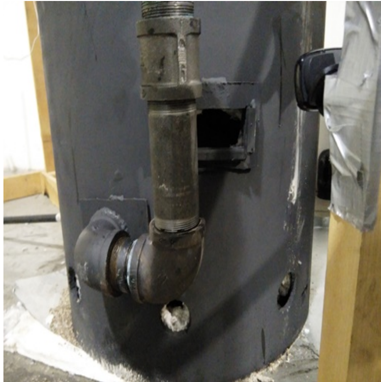
Figure 2.6. Combustion flare showing camera, window flame and air holes
