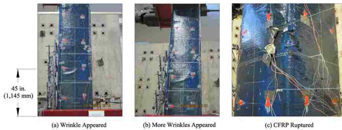
Fig. 5 - Failure of repaired column.
