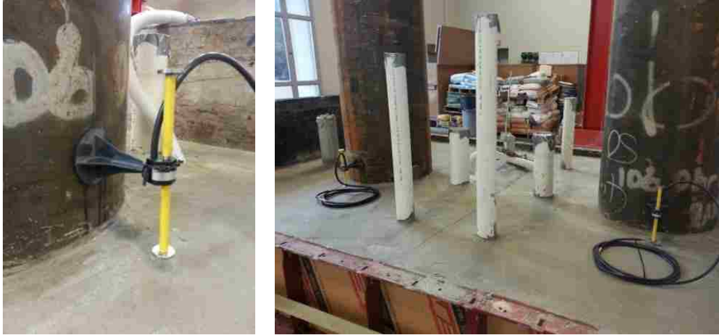
Figure B.14. Install vibrating wire strain gauges in the concrete wall thickness
