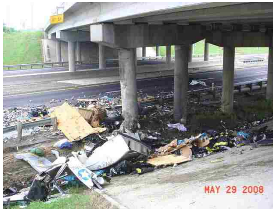
Figure 2.7. Truck-tractor-trailer accident–FM 1401 Bridge, Texas, 2008 (Buth et al. 2010)
