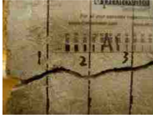
Figure 2.7 Typical corrosion-induced cracks on the concrete surface with a crack meter.
