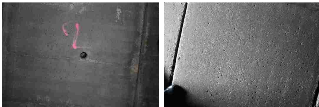
The cracks on the top (left) and bottom (right) of Box 16
