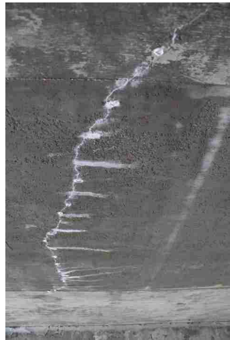
Figure 5.19. The cracks of span 6
