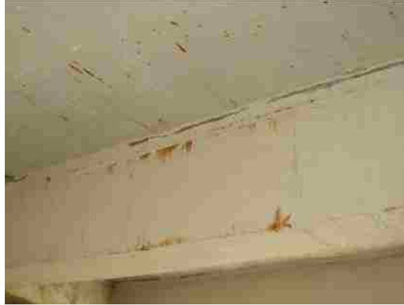
Figure 4.1. Corrosion of a transverse girder of Bridge P-0926 [23]
