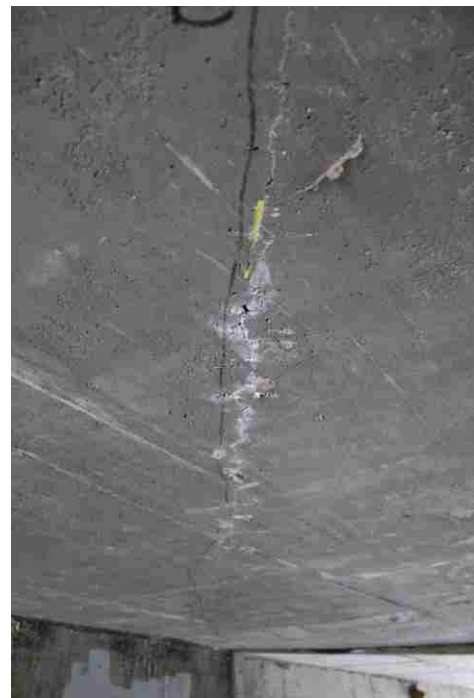
Figure 5.15. The cracks of span 2
