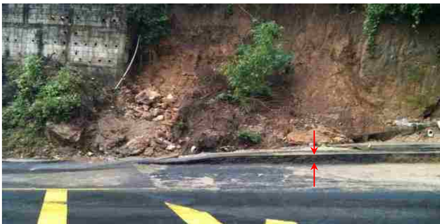
Figure 3.7. Ground heave due to active landslide
