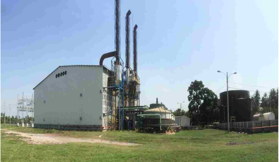
Figure 4.35. Panoramic view of Genosa Power Plant
