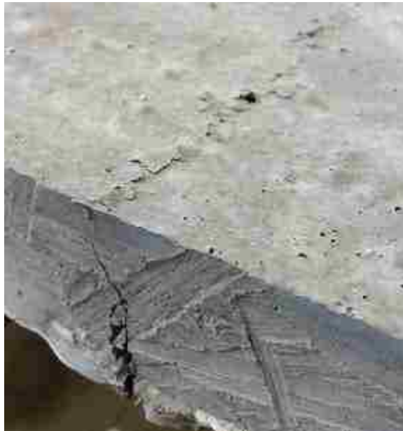
Figure 6.55. Tensile crack on panel SUN2
