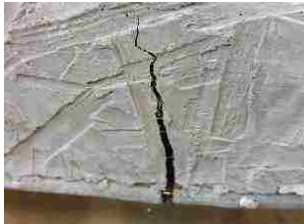
Figure 6.10. Tensile crack on panel FUC3
