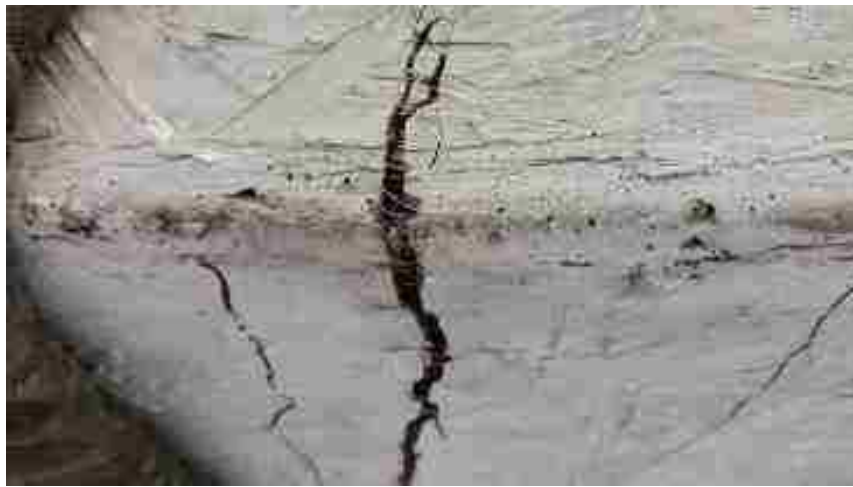
Figure 6.44. Tensile crack on panel SUN3
