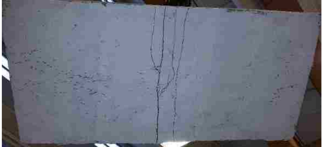
Figure 6.27. Crack pattern formation at the tension face of panel FUN2
