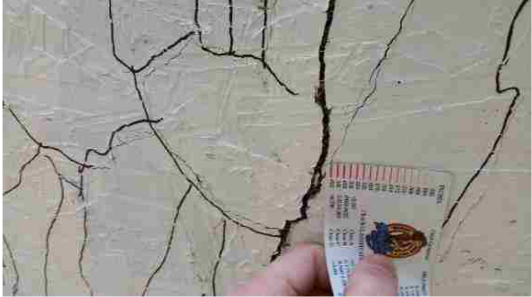
Figure 6.51. Crack widths at the tension face of panel SUC2
