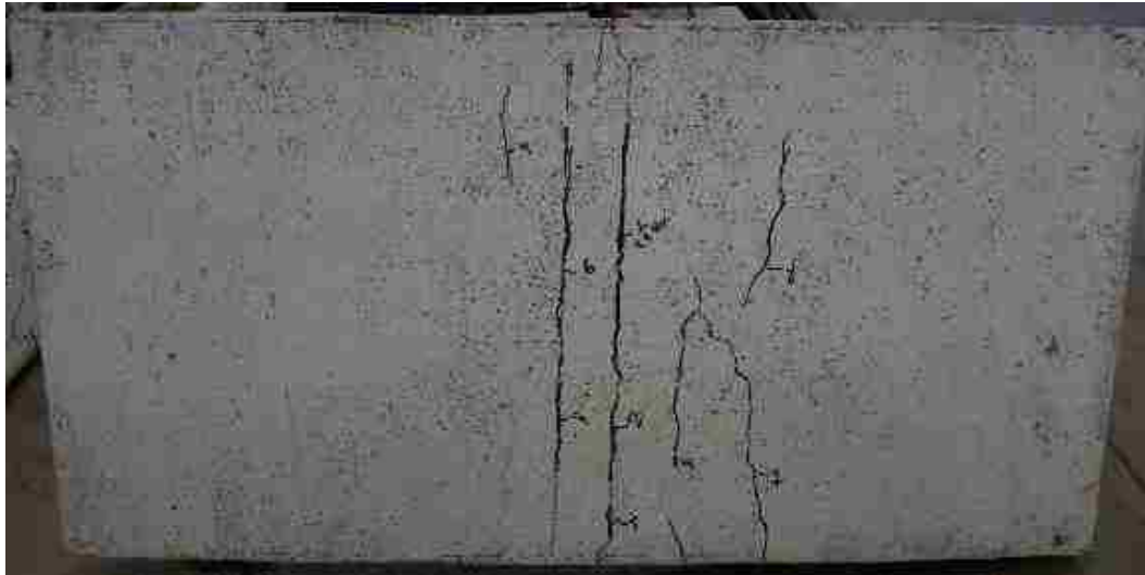
Figure 6.2. Crack pattern formation at the tension face of panel FCC3
