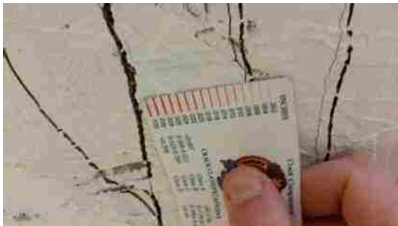
Figure 6.28. Crack widths of panel FUN2
