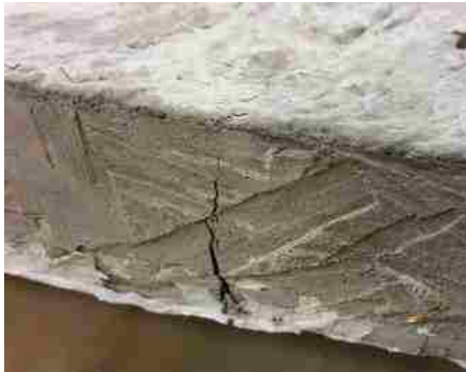
Figure 6.26. Tensile crack on panel FUN2
