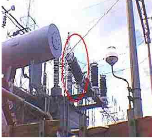
(a) Broken Bushing of a Transformer
