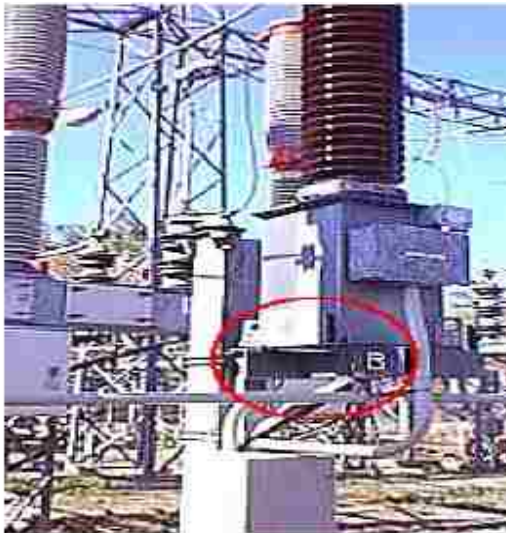
(c) Oil Leakage from the Bottom of Radiator
