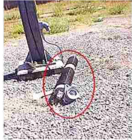
(b) Broken Bushing of a lightning rod
