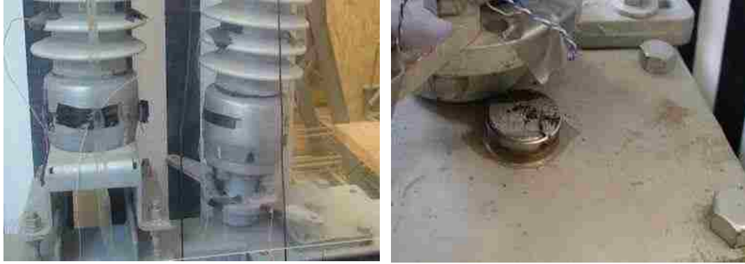
Figure 7.14. Fracture Detail and Failure Location
