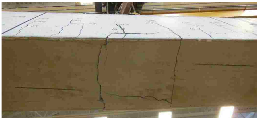
Figure D-20. Crack Pattern of Specimen BWOC-70 (Bottom View)
