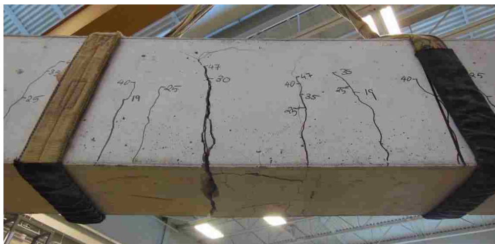
Figure D-14. Crack Pattern of Specimen BWC-60 (Bottom View)
