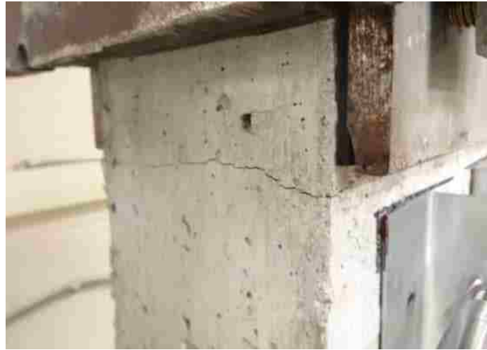
Figure 3.27 Typical Hairline Flexural Flange Crack Observed In Shale Aggregate Concrete Specimens
