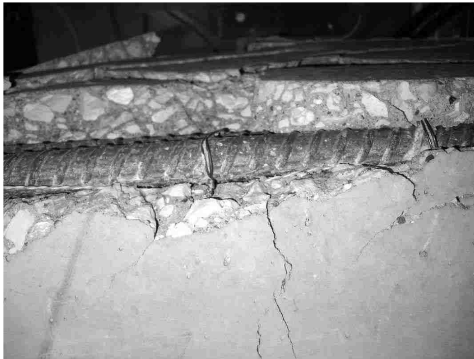
Figure 5.4. View of Black Rebar in Splice Region of Beam 6B32N
