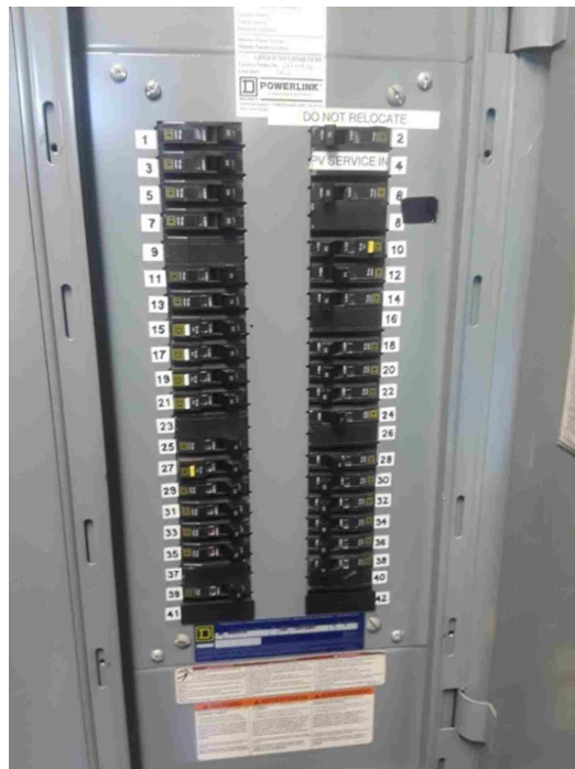
Figure 3.13. Chameleon home circuit panel
